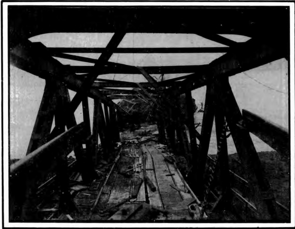
View of collapsed north span with north pier in the distance.
