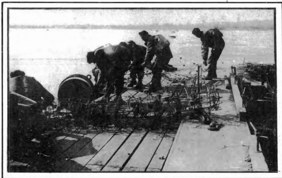
Attaching mine net to jackstays showing net being unrolled across bow of infantry support raft and intermediate float and net weights attached.
