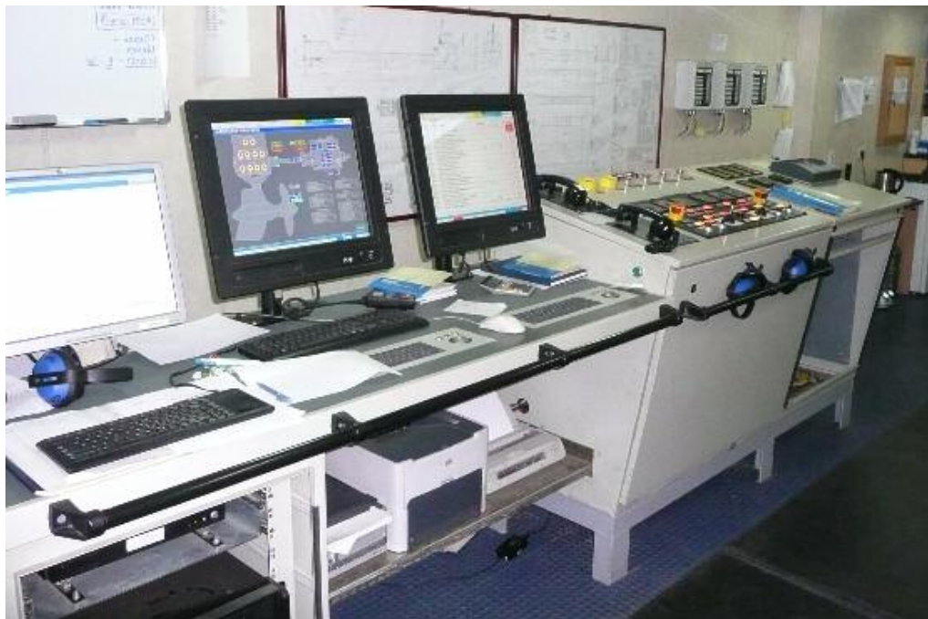
The Engine control room
