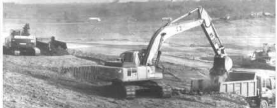
The construction site of Ma Mya Dam Project being implemented by Construction (9) of the Irrigation Department under the Ministry of Agriculture and Irrigation.
