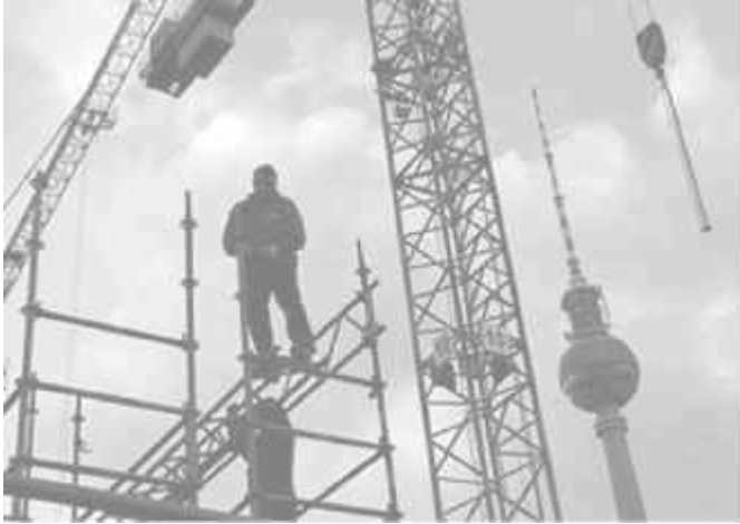
Workers at a construction site in Berlin's Alexanderplatz square. Business confidence in Germany rose to its highest level in 15 years in April, underlining the robustness of the ongoing recovery of Europe's biggest economy.—INTERNET
