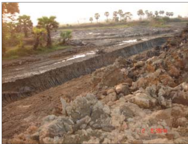
Land Was Destroyed by Water Flow Canal
