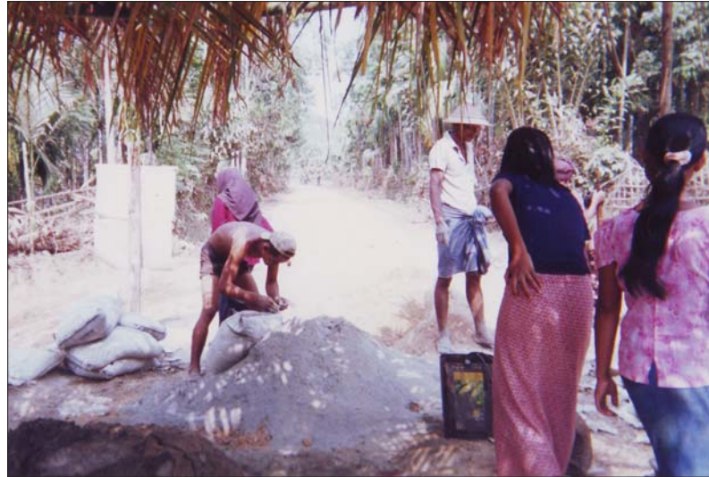
Civilian Piling cement for building the bridge in Development project in Khaw-Zar
