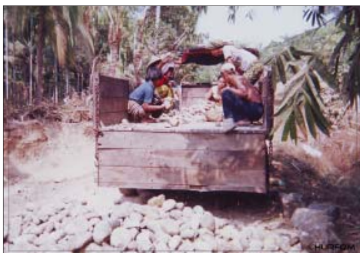
Villagers, included women were forced to carry rock to repair the Khaw zar - Magyi road. Photo No.2
