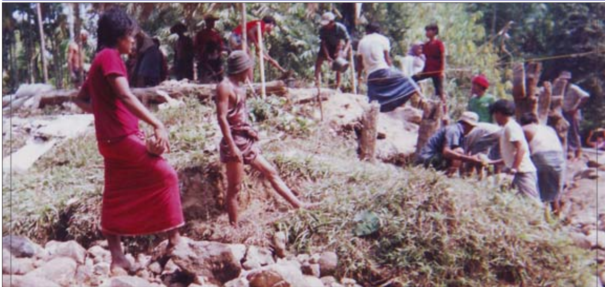
Forced labourers in a bridge construction near Yin-Ye village, Ye Township, Southern Mon State. (photo:HURFOM)
