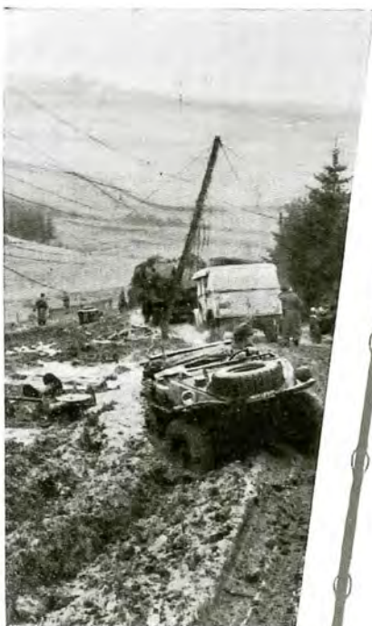
This is rough on cable crews
