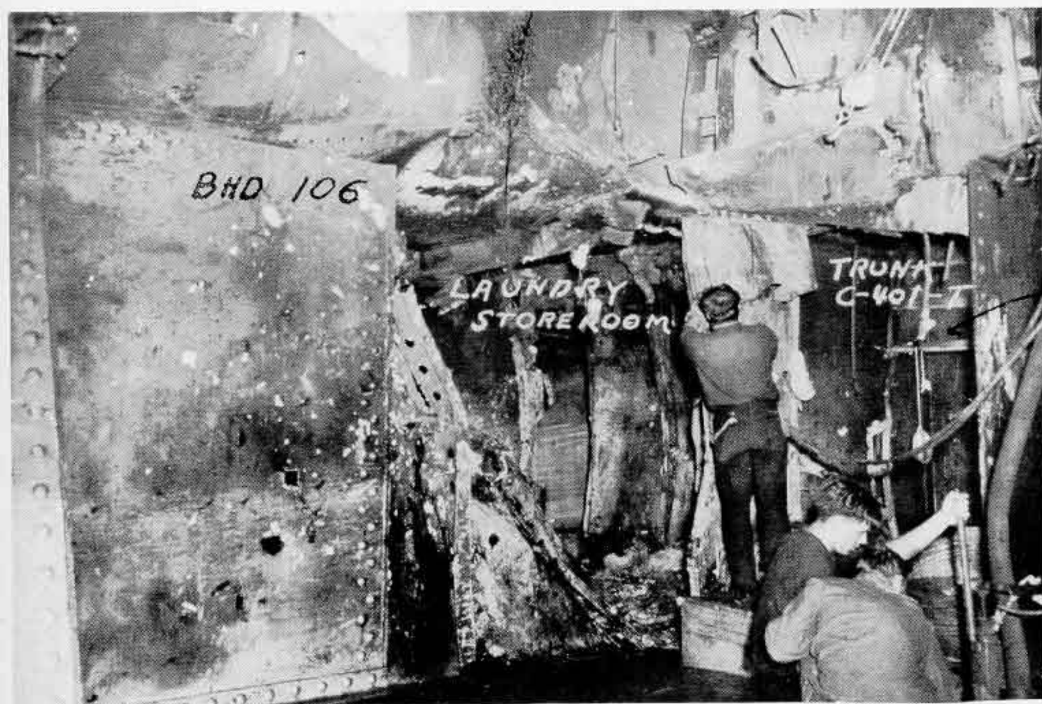
Photo 18: Damage on 4th deck, looking forward and to starboard. Note inboard longitudinal bulkhead of trunk C-401-T has been blown out. Laundry storeroom is forward of hole in bulkhead 106.
