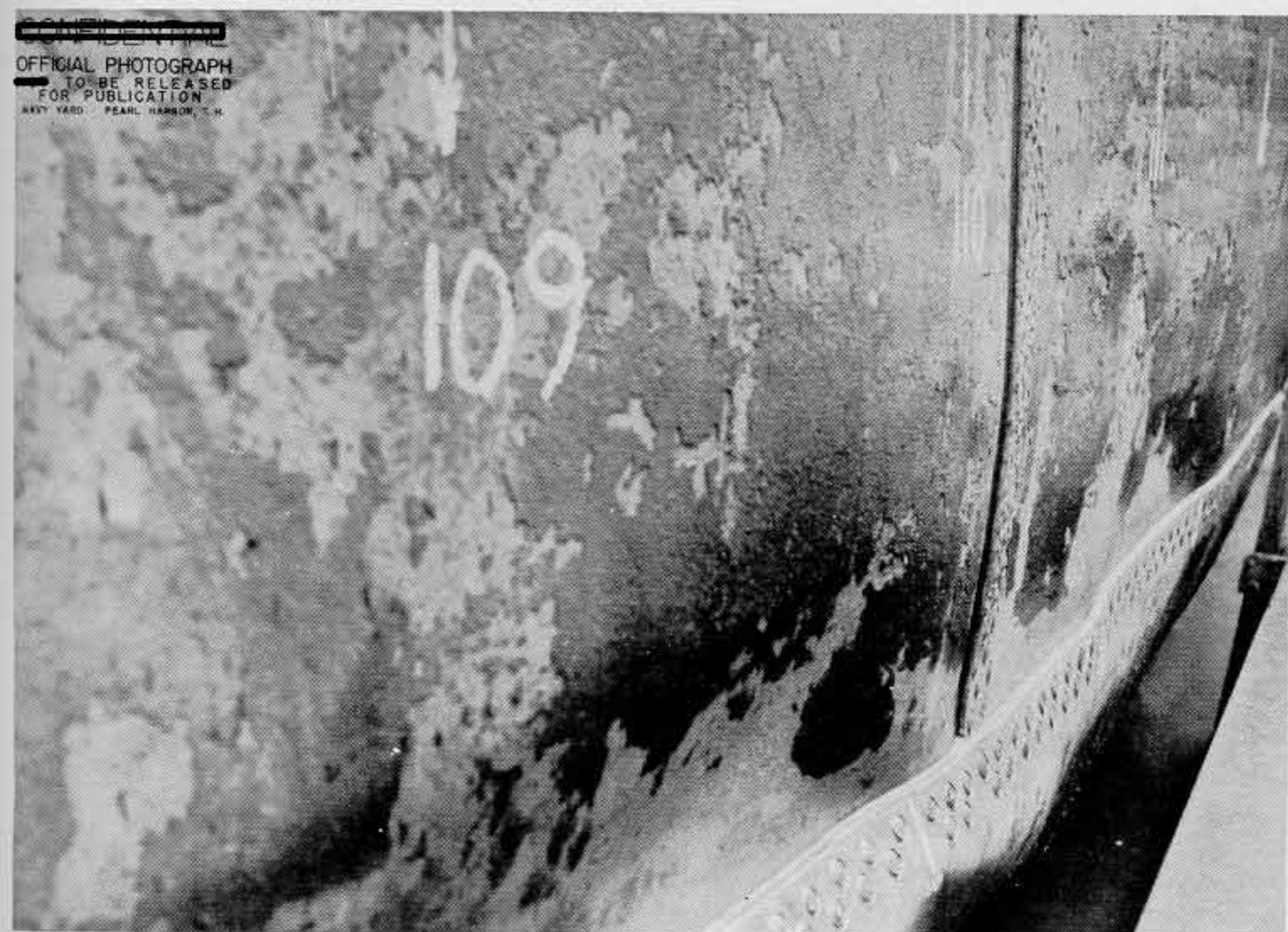
Photo 1: Bomb Damage to Port Shell, looking aft, FRS108-112.
