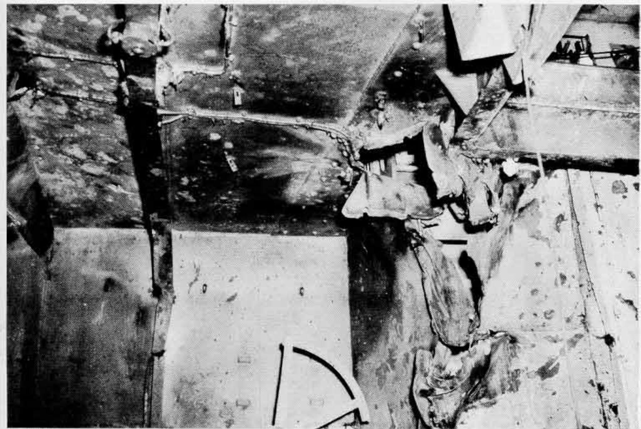
Photo 10: Bomb Hole, Second Deck, FR 107, looking forward and up. Note after inboard corner of transverse access trunk C-501-3T which deflected bomb inboard.
