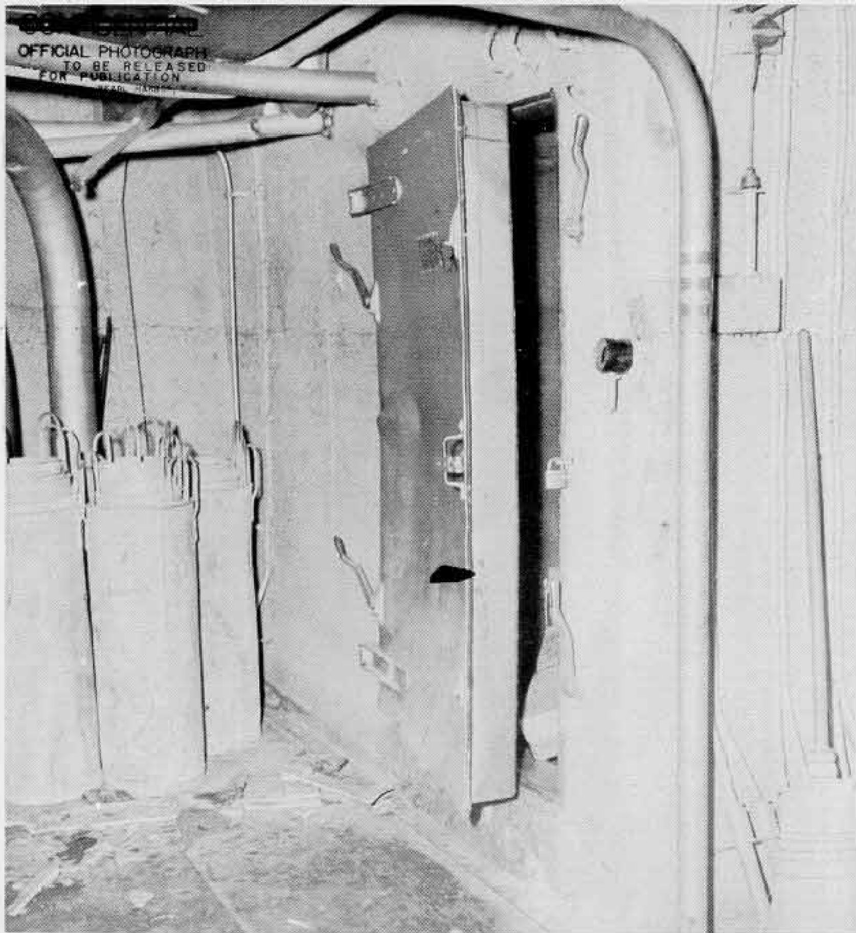
Photo 27: Refrigerator door, 4th deck, 13'-0" to starboard of centerline, FRS 127-129. Note deflection. This was 80' aft of explosion.
