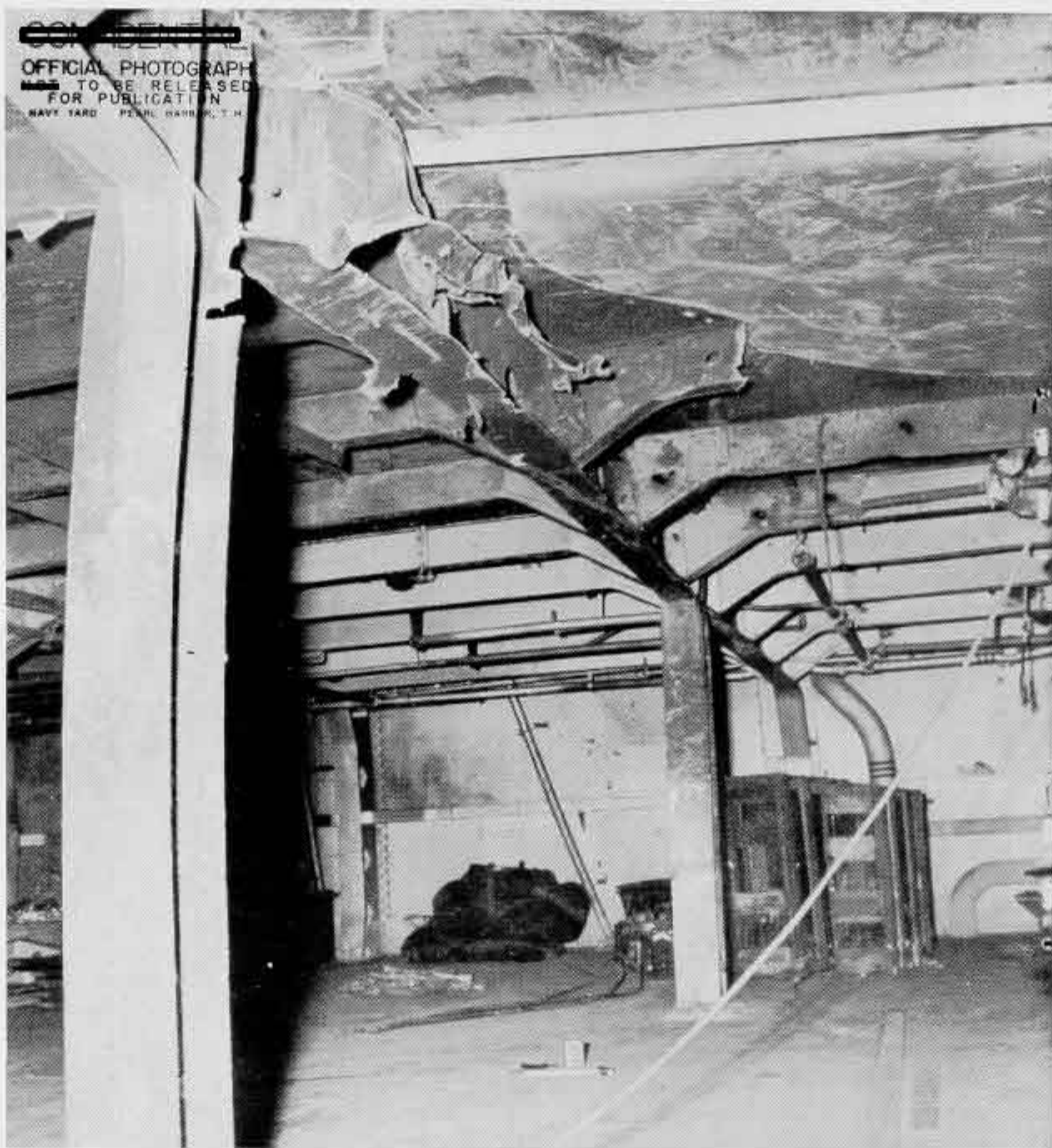
Photo 19: Web FR 109, underneath 3rd deck, looking to port.
