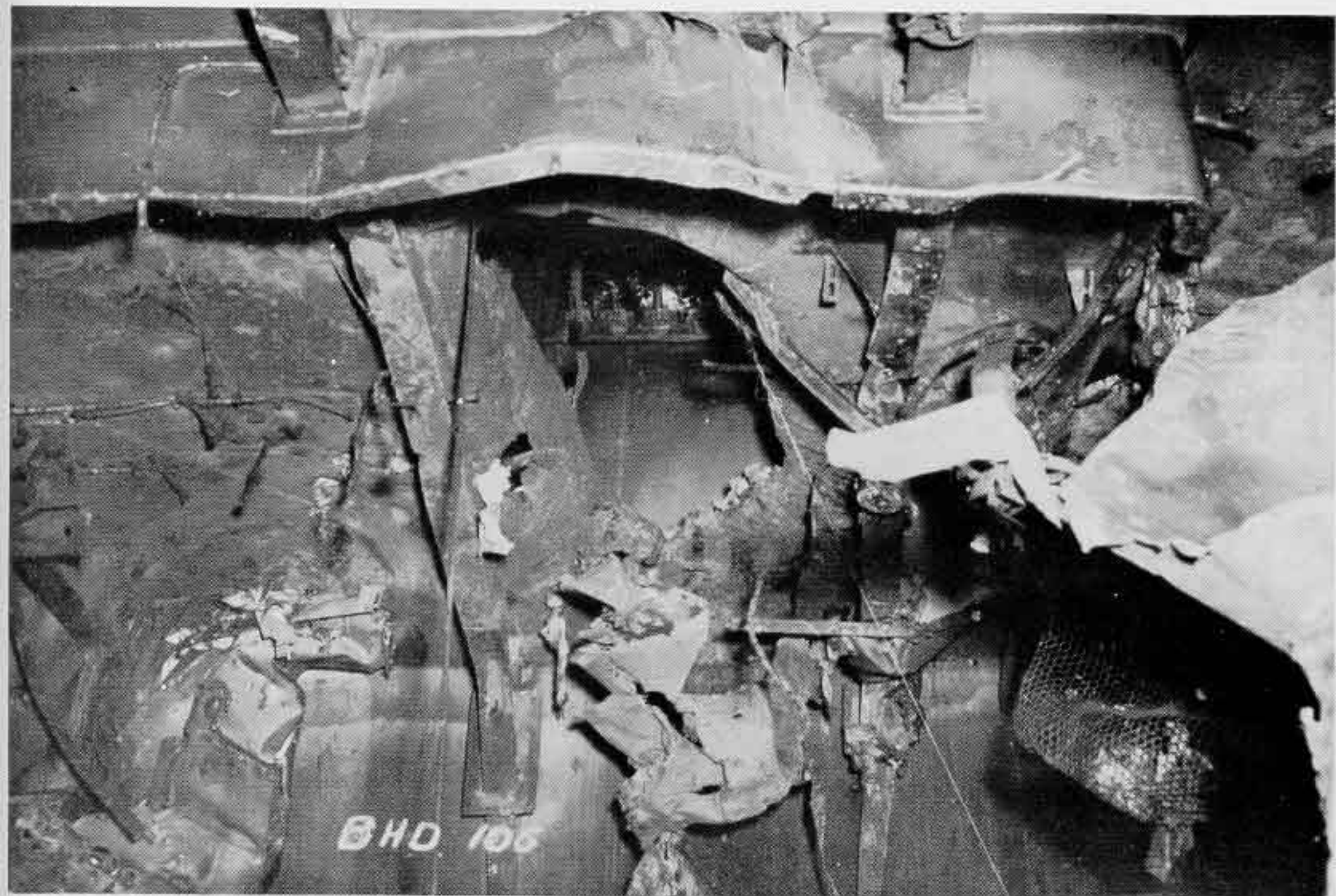
Photo 26: Bomb blast hole, second deck, FRS 106-107, starboard.
