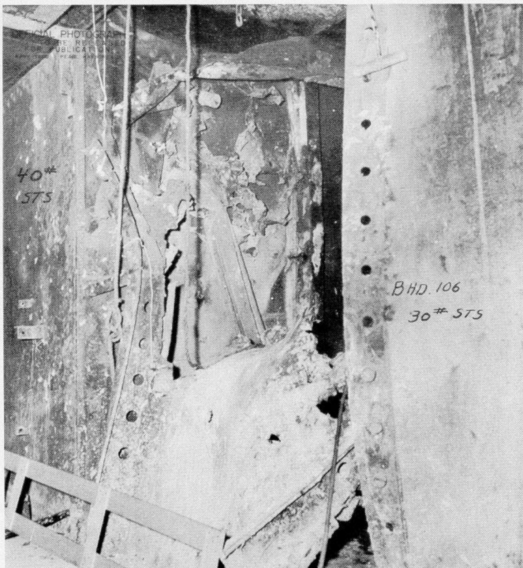
Photo 15: Damage to Bulkhead 106, between 4th and 3rd decks, looking forward and inboard.
