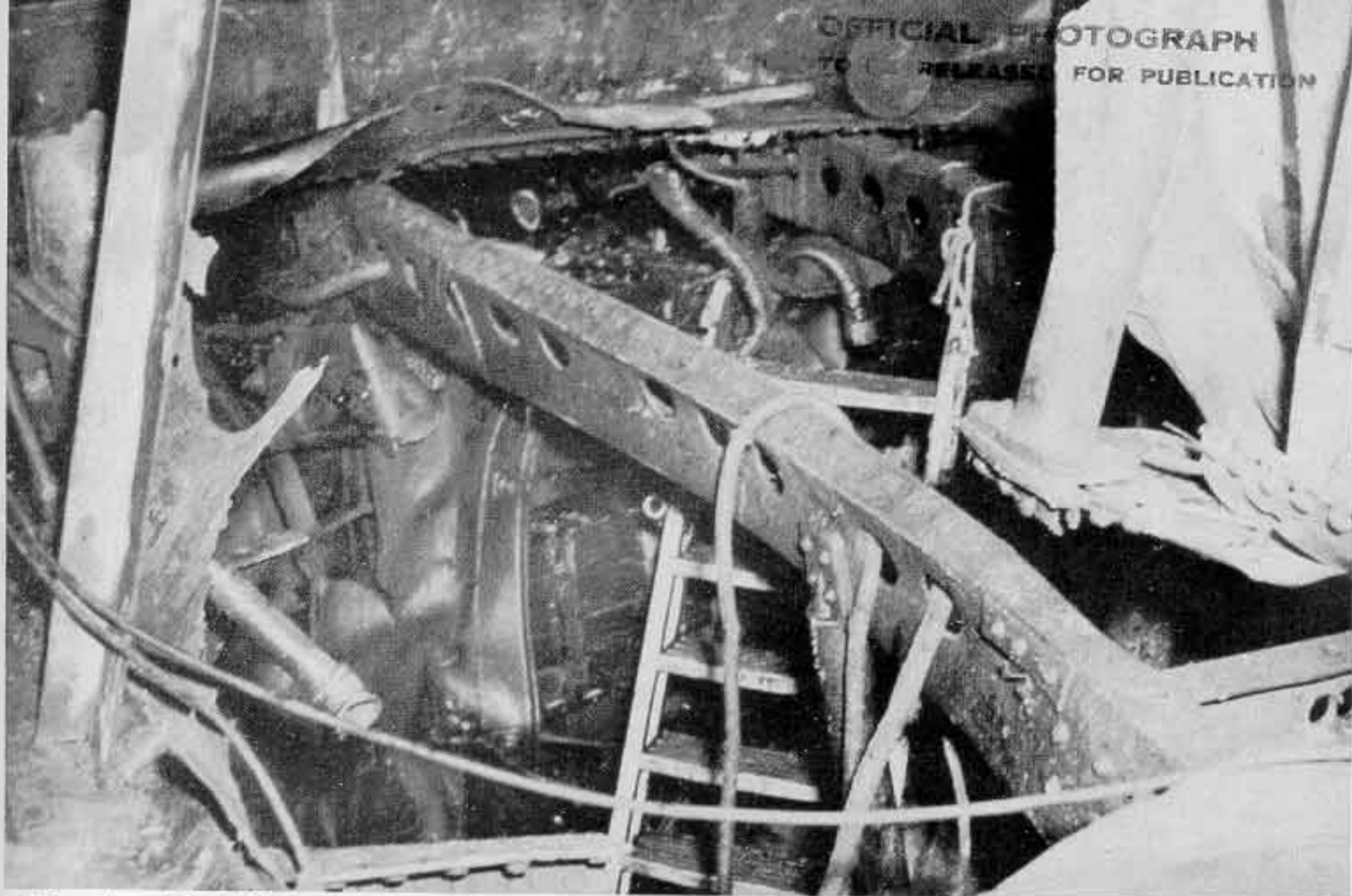
Photo 7: Hole in first platform deck frames 125 to 127 portside.
