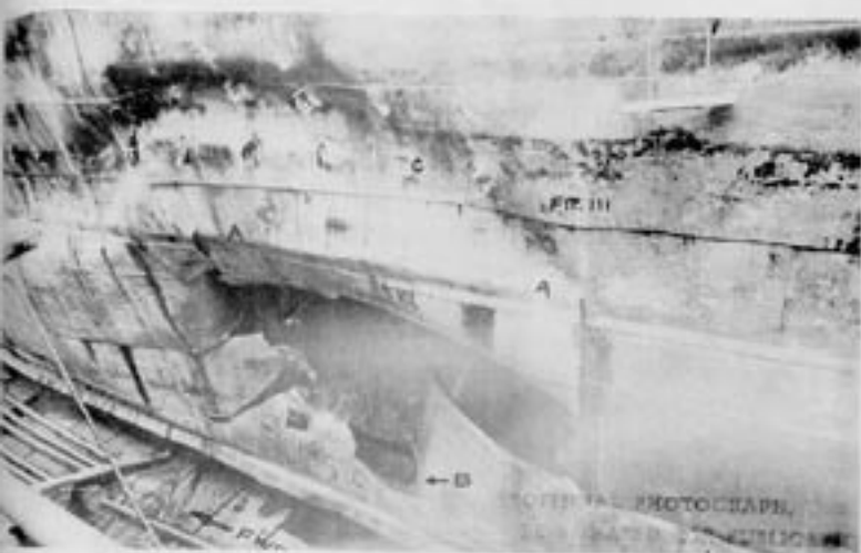
Photo No. 2: View from half-way down the dock, looking forward. Countersunk rivets pulled out at B. Channel struts in upper blister pierced the plating, as at C.
