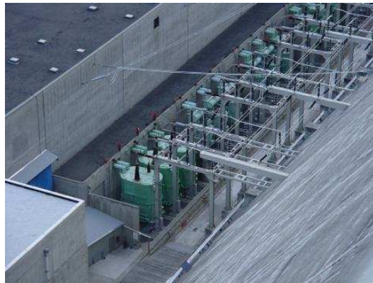
Figure 10.48: Step-up transformer bank at Grand Coulee hydroelectric dam, Washington state, USA.
