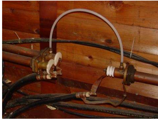
Figure 14.52: Flexible coaxial cables connected to rigid lines.
